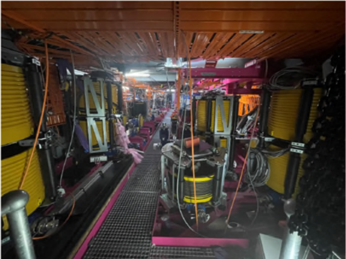
Plate 7: Technical Zone: Winch Installations
