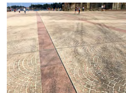
4.462 Adhesive remains before cleaning, 2016
